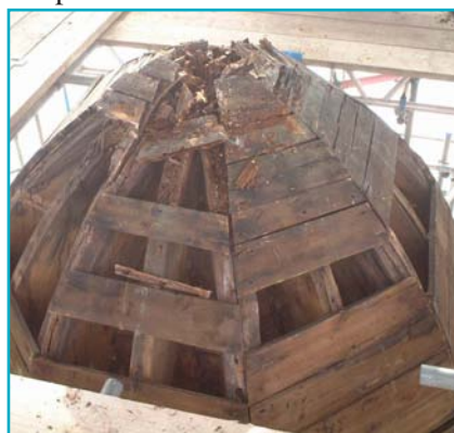
Decayed timber at the top of the Cupola
